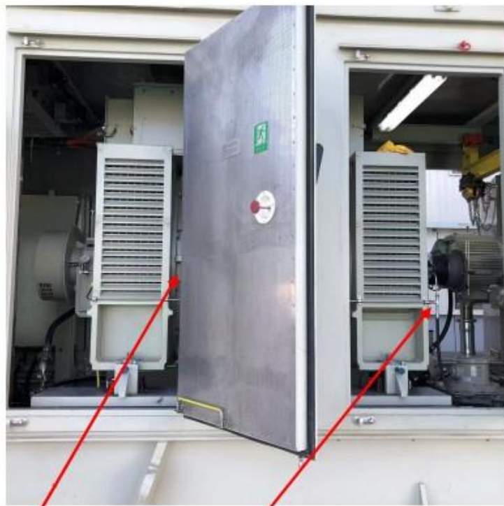
Generator+generator lubricating oil pipeline
