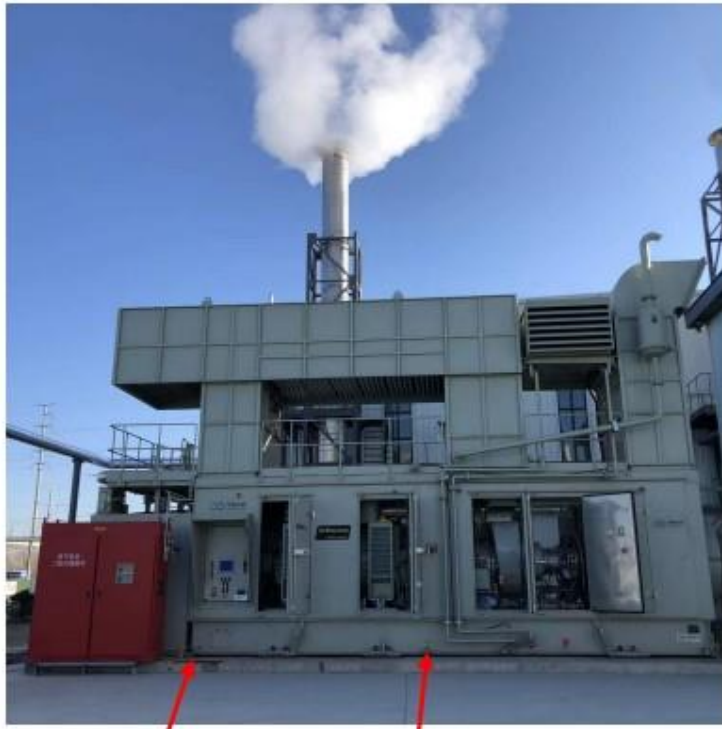
Low level oil discharge port of turbine lever+oil tank discharge port
