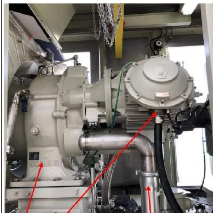
Gearbox+starter motor junction box+oil pump outlet pipe
