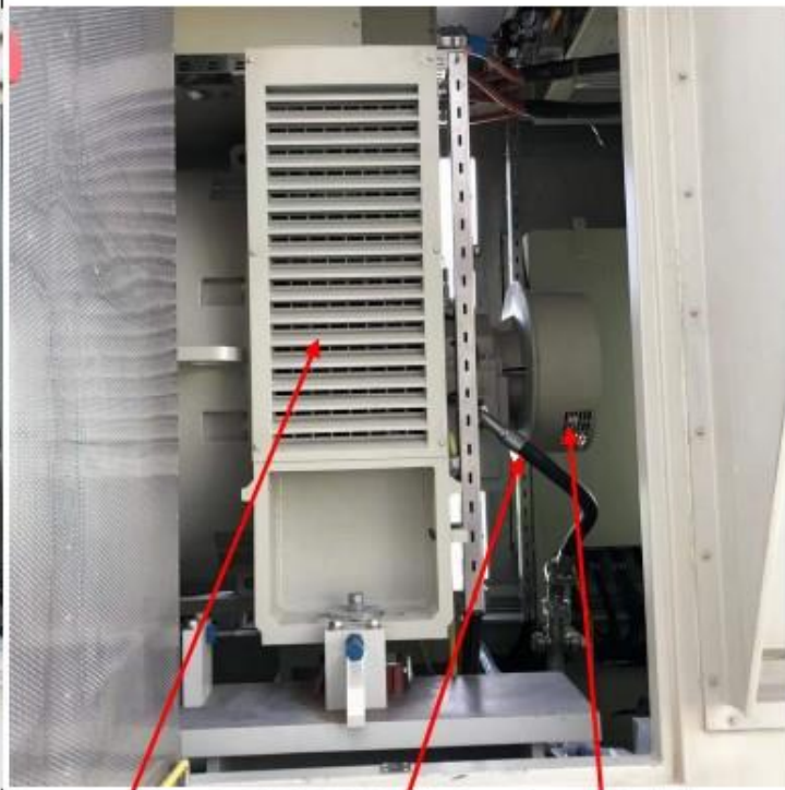
Generator cooling air outlet+lubricating oil return pipe+rectifier bridge
