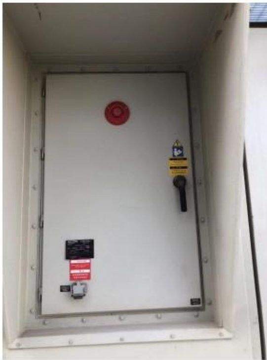
JB72 Generator Control
