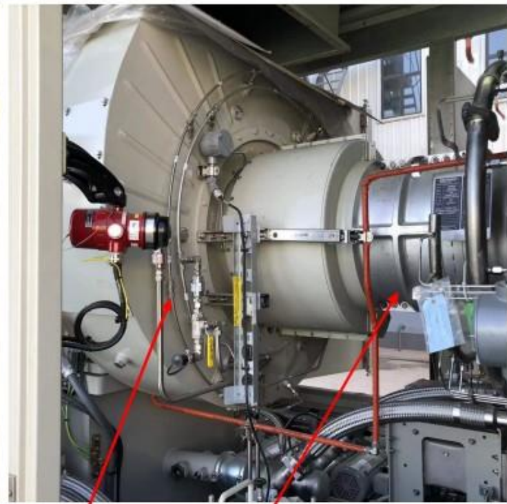
Gas turbine cleaning nozzle pipeline+compressor (12 stage stationary and moving blades)
